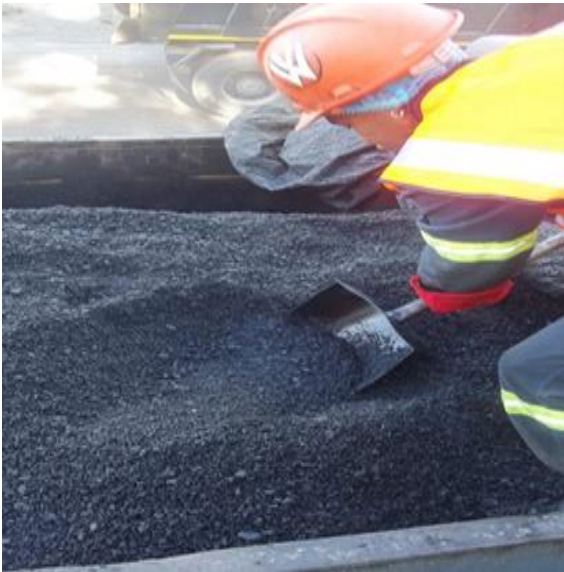
Figure A4: Setting the Crust of the Asphalt Aside and Digging into the Pile
