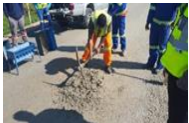
Figure A9: Using a Pick to Loosen the Material and Dig through the Entire Layer
